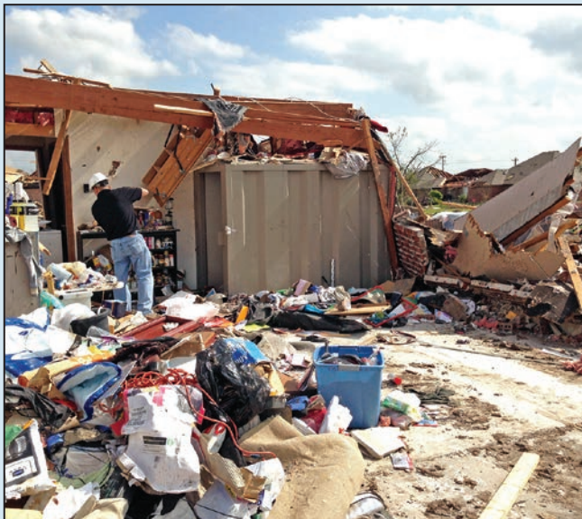
Above-ground shelter that performed well in a heavily damaged area (Oklahoma City, OK, 2013)
