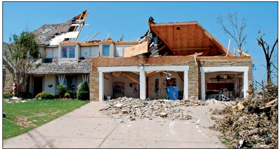
Figure 2-7: Example of a garage door failure that likely initiated progressive failure, including loss of the garage roof (Joplin, MO; EF2 rating per MAT investigation)
