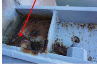
Photo 36 – Pier 3, left trunnion for gate 1. Failed casting is leading to corrosion on the web and stiffener plate. Metal loss on these components appears to be significant. This condition is typical of all the trunnions.
