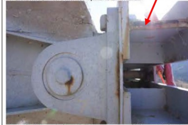
Photo 40 – Pier 9, left trunnion for gate #7. The next two photos are taken between the horizontal anchor girders.
