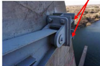
Photo 35 – Pier 3, left trunnion for gate 1. The next two photos show extensive corrosion on the web of the anchor girder.
