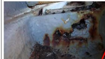
Photo 39 – Pier 6, left side of the trunnion, bottom horizontal girder, viewing the stiffener on the top of the web. Extreme section loss due to corrosion was present on this web stiffener.
