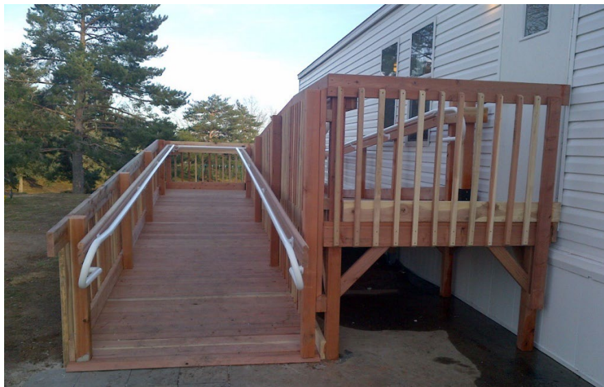
Figure 6: An example of a FEMA manufactured home used in Colorado. This home had a ramp added to make it accessible for a wheelchair user. FEMA Photo
