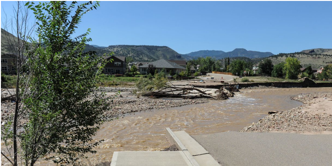
Figure 8: Restoring McConnell Drive was one of the largest Public Assistance projects in Lyons. FEMA Photo
