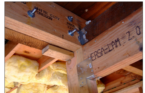
Structural Risk: A homeowner retrofitted their home with earthquake straps and bolts to prevent movement in the event of an earthquake.
