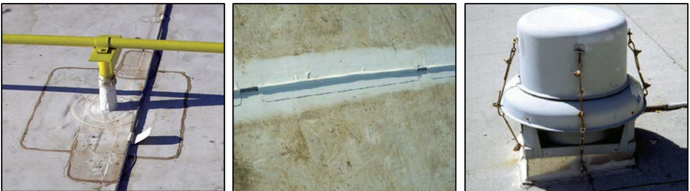
Figure 3.3.2.5. Rooftop periodic gas line supports using a steel angle welded to a pipe that was anchored to the roof deck for lateral and uplift resistance (left). Use of intermittent membrane flashing to secure a lightning protection system conductor (center). Cables attached prevent rooftop equipment cowling from blowing off (right).
