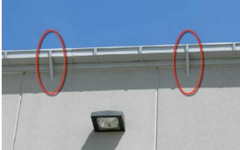
Figure 3.3.1.10. Sheet metal straps (circled) attached to an existing gutter to increase wind uplift resistance.
