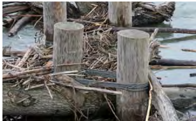
The timber piling structures capture woody debris, which provides roughness to the river, and ultimately establishes additional habitat.
