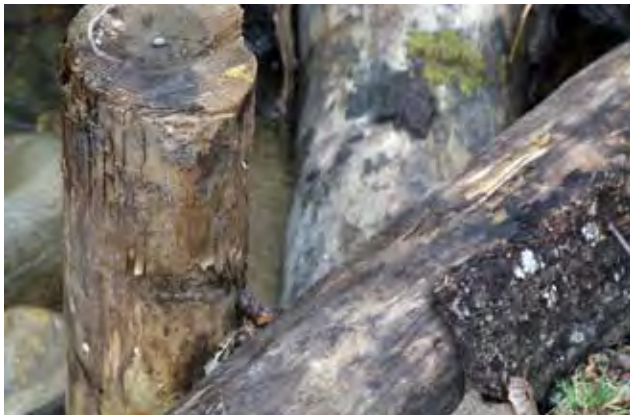
The logs in the jams are secured to each other with rebar.
