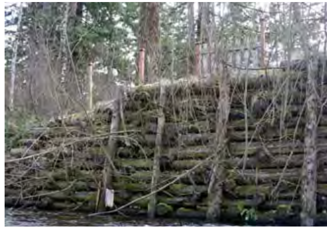
The crib wall will overgrow with vegetation, which will ultimately become the structure itself when the logs finally decay.
