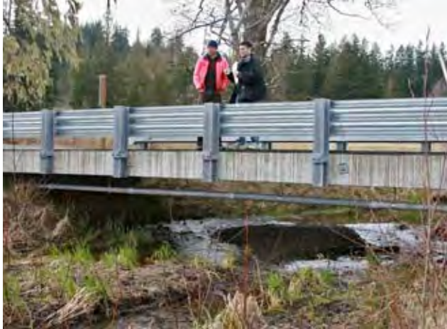
The extra wide design of the bridge ensures adequate room for water flow during flood conditions.
