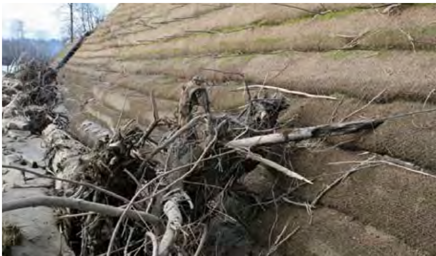
The offsetting of the soil wraps comprising the structural earth wall (SEW) give it its step-like appearance. The logs anchored to the toe of the embankment protect the structure from fast flowing woody debris and provide habitat for migrating fish during high water.
