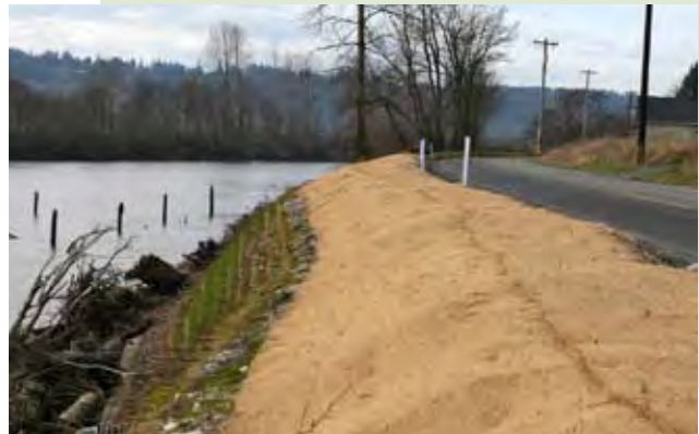
Eventually the coir fabric and the structural earth wall itself will be completely overgrown with hydro-seeded grass and other vegetation.
