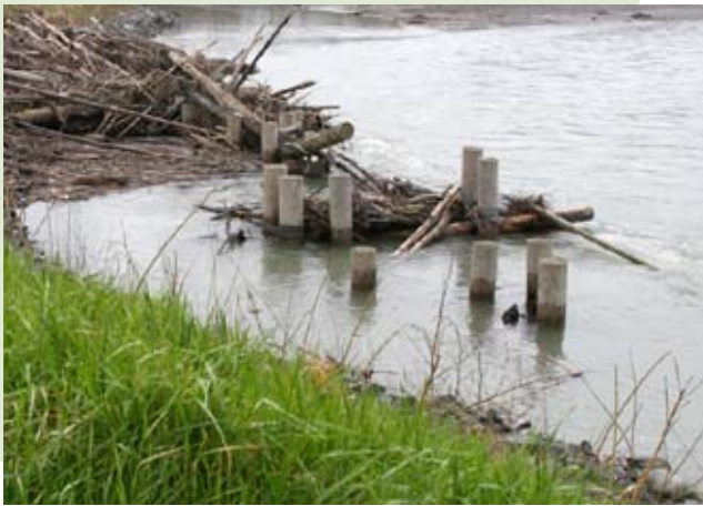
One of the scour holes being stabilized by the Overflow project. Woody debris has begun to collect and will be incorporated into the riverbank.
