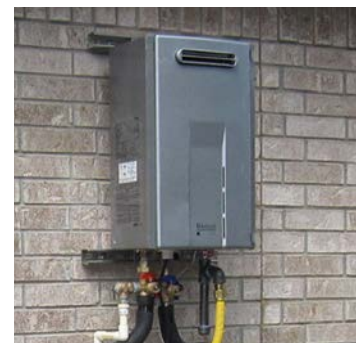
▲ Tankless water heater affixed to a building servicing the insured property.
