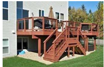
▲ A deck with two sets of stairs; only one is covered for egress.
