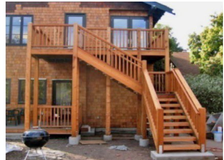
▲ A deck with a single set of stairs providing access to the building through two doors.
