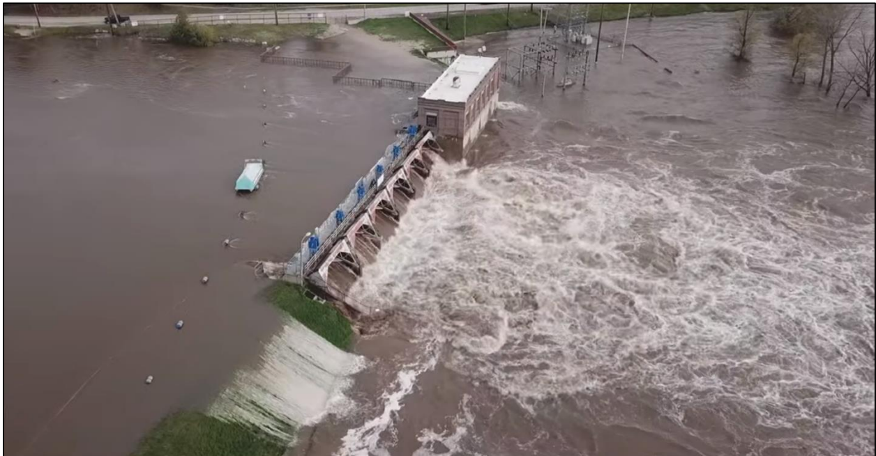
Figure 9: Sanford Dam overtopping on May 19, 2020 (CFI Media 2020)
