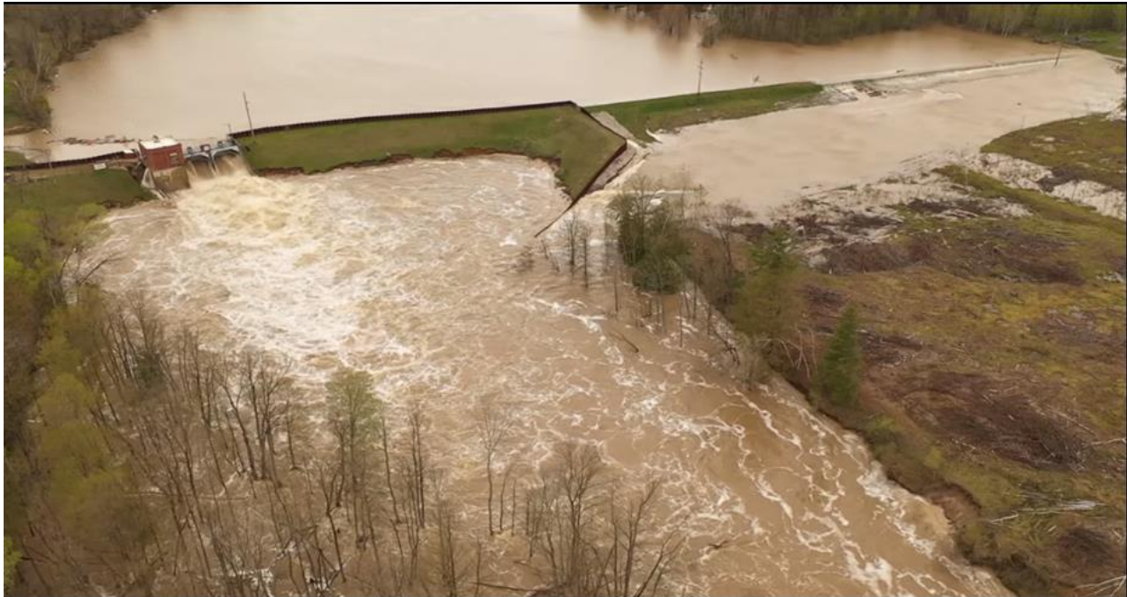
Figure 6: Smallwood Dam erosion and emergency spillway activation during the May 2020 flood event (Jacuzzibusguy 2020)
