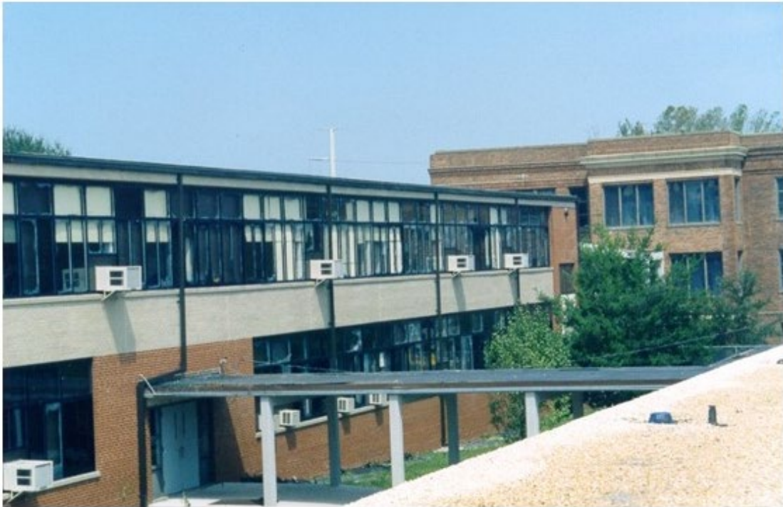
B) Significantly Less Windows Damaged on the Lower-Right Glazed Area than on the Upper Glazed Area
