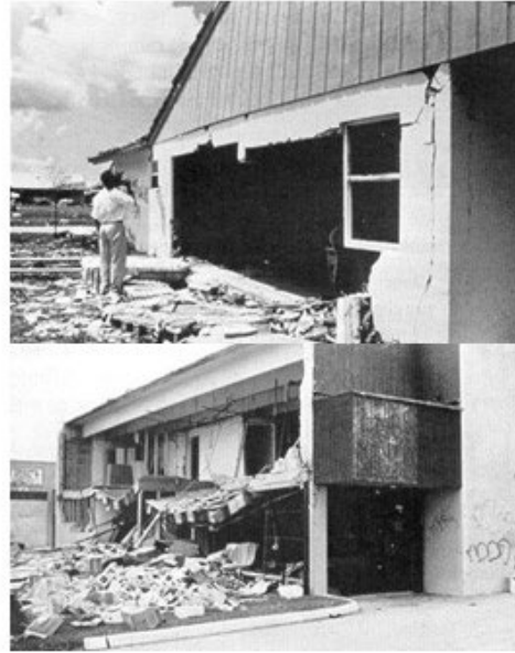
B) Collapse of masonry walls (Zollo, 1993): (top); A wall of 40' span Walls on a two-story building (bottom)
