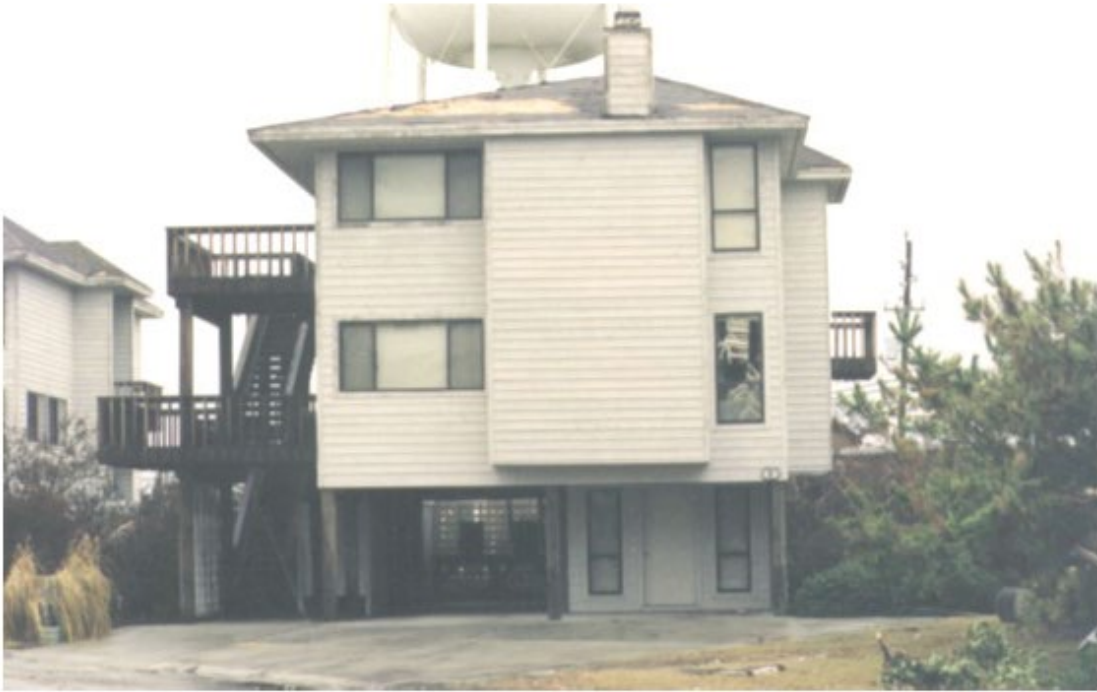
A) 2% to 15% Roof Cover Loss, One Broken Window
