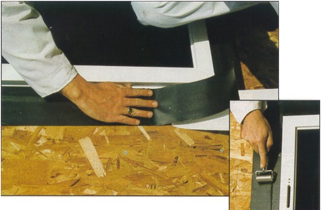
Figure 8-15 Example of Self-Adhering Waterproof Underlayment Used to Tape Plywood Joints, Ridges and Eaves; Photo Depicts Use Around Fenestrations
