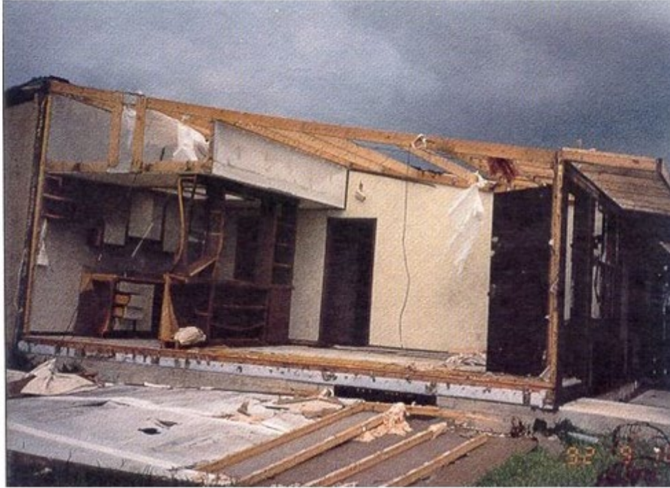
C) End wall separated from end unit of a modular home
