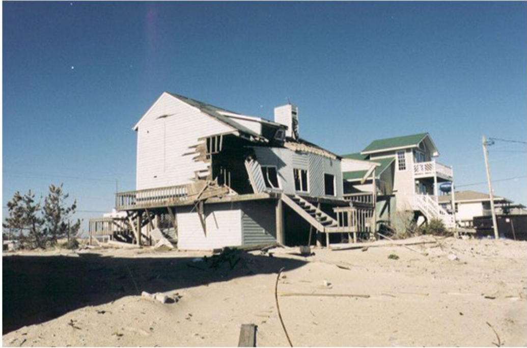
C) Wall Failure
