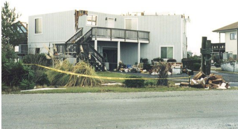
A) Complete Roof Failure
