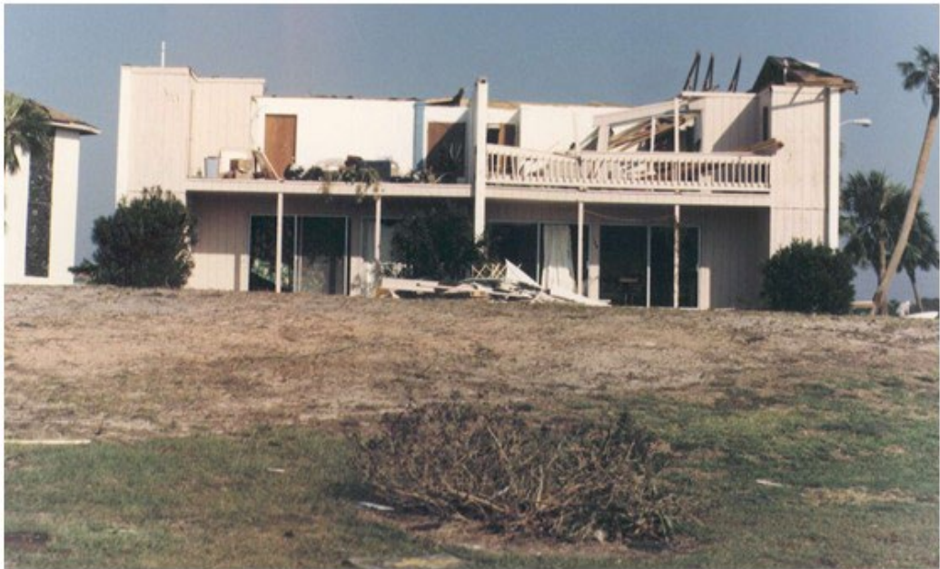
D) Whole Roof Failure, Wall Failure
