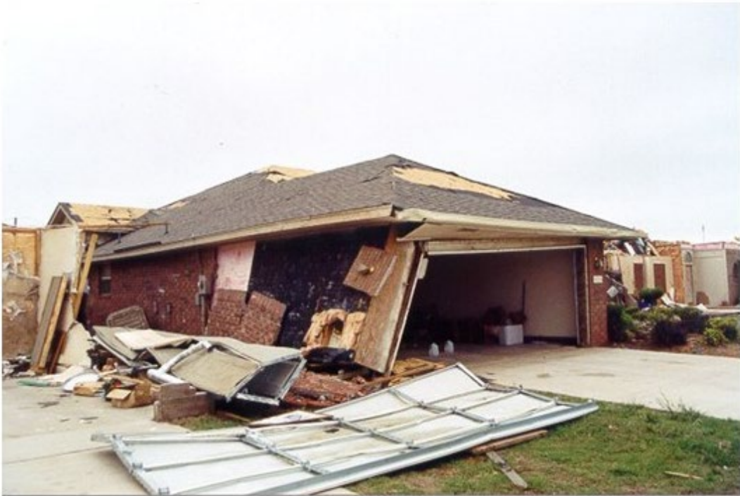
B) A wall section collapses
