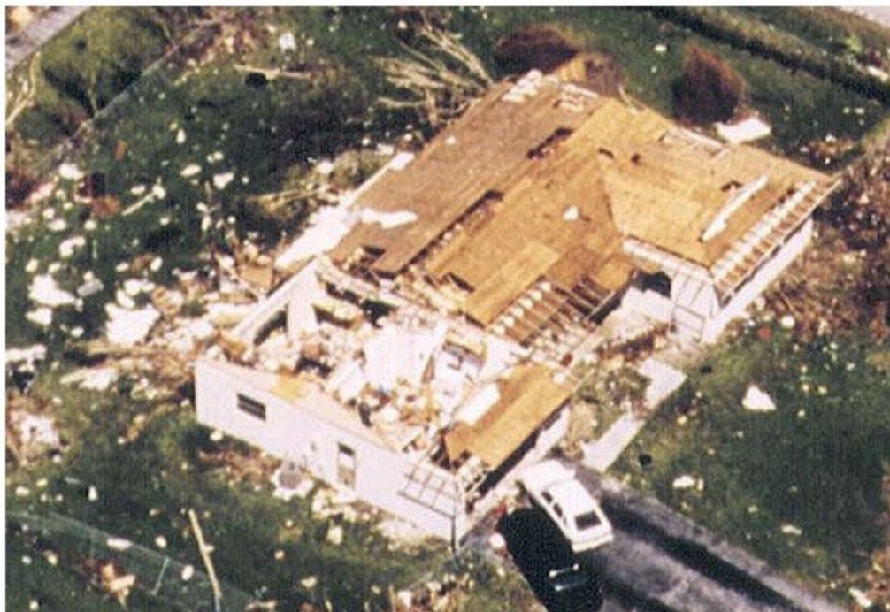
B) Complete Roof Failure, Greater than 25% Sheathing
