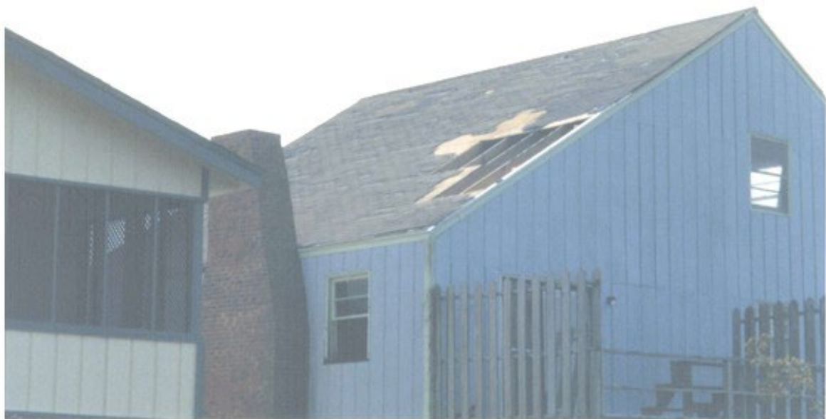
B) At least One Failed Sheathing but Less than Three Failed Pieces of Roof Sheathing
