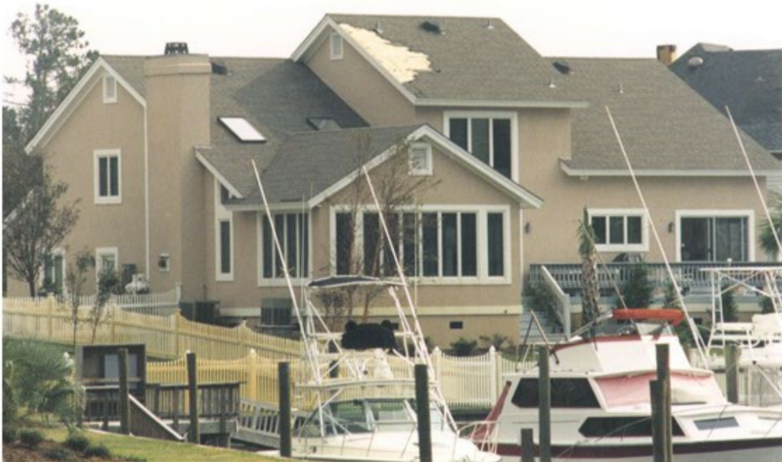
B) 2% to 15% Roof Cover Loss
