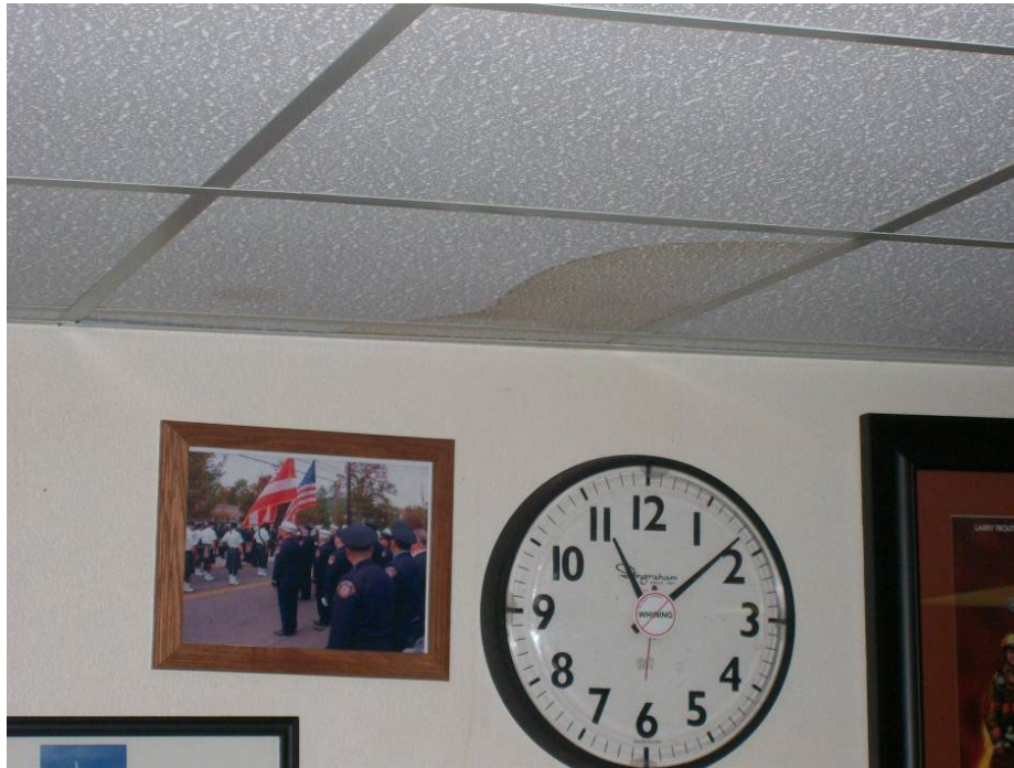
Figure 5-145 Water Damage to Interior Ceiling of a Fire Station in the Houston Area as a Result of Roof Damage (2008, Hurricane Ike)
