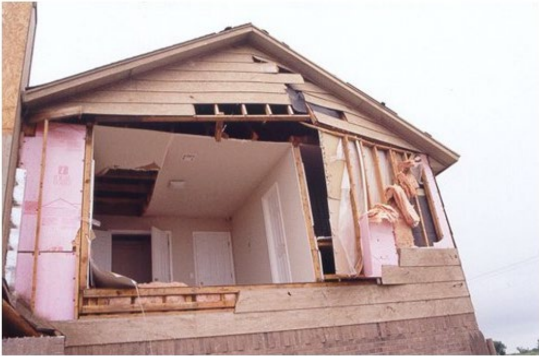
A) Exterior wall fails in sections at connections to other parts of the structure
