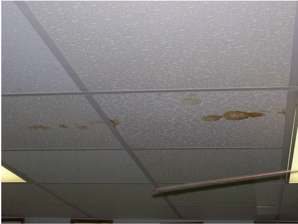
Figure 5-145 Water Damage to Interior Ceiling of a Fire Station in the Houston Area as a Result of Roof Damage (2008, Hurricane Ike)
