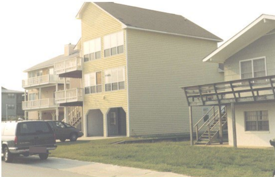
D) One Broken Window
