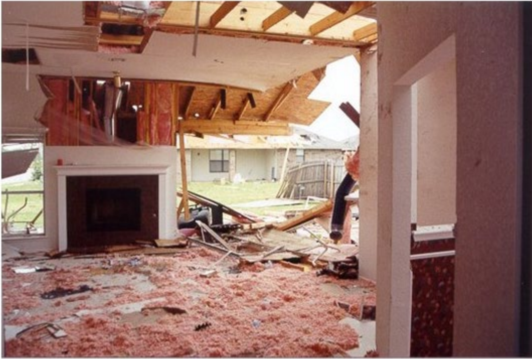
A) Garage wall fails at the connections to the foundation
