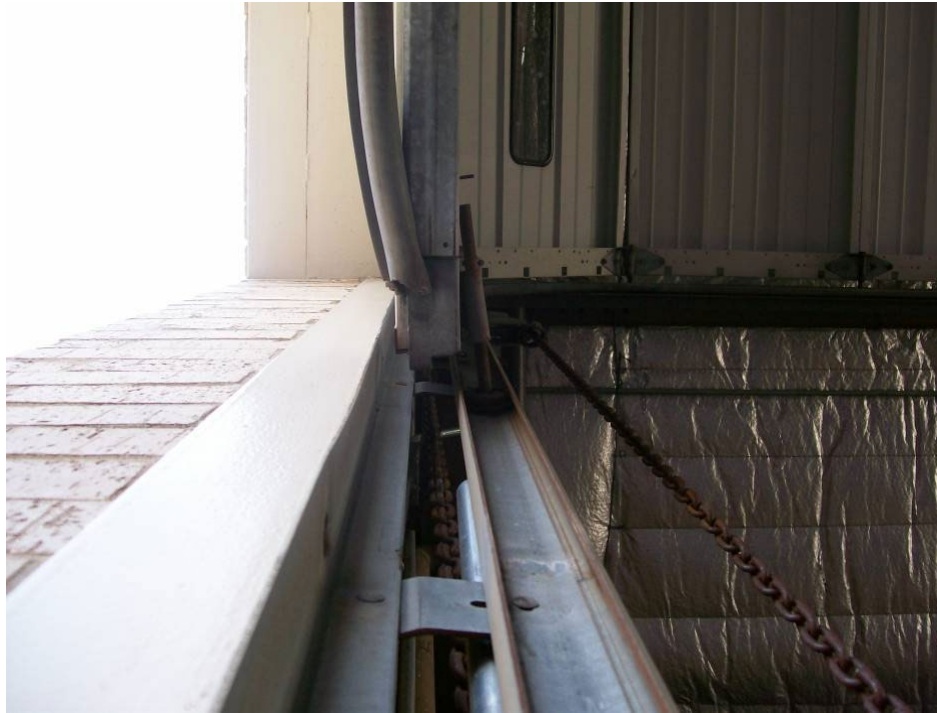
Figure 5-146 Bent Bay Door Rollers for a Fire Station in the Houston Area (2008, Hurricane Ike)
