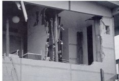
D) Collapse of masonry wall (HUD, 1993)
