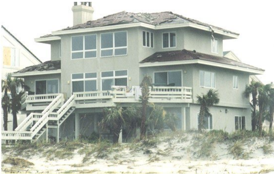
C) 2% to 15% Roof Cover Loss
