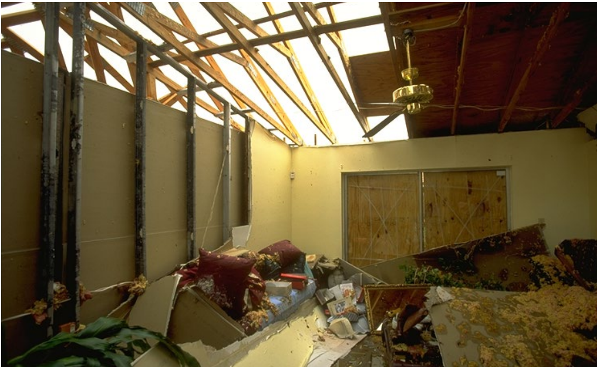
Figure 8-3 Content and Interior Losses Associated with Roof Sheathing Failure
