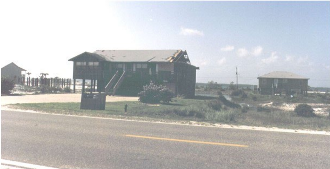
More than Three Pieces of Failed Roof Sheathing but Less than 15% of the Panels Missing
