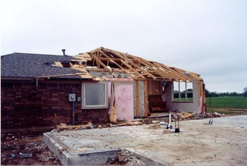
B) Wall failure while roof frame still in place
