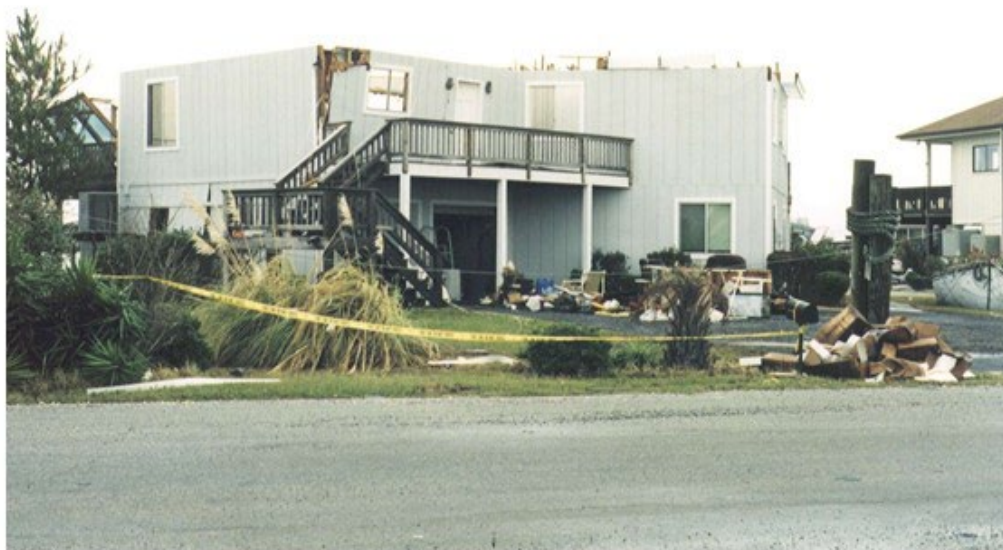
A) Complete Roof Failure
