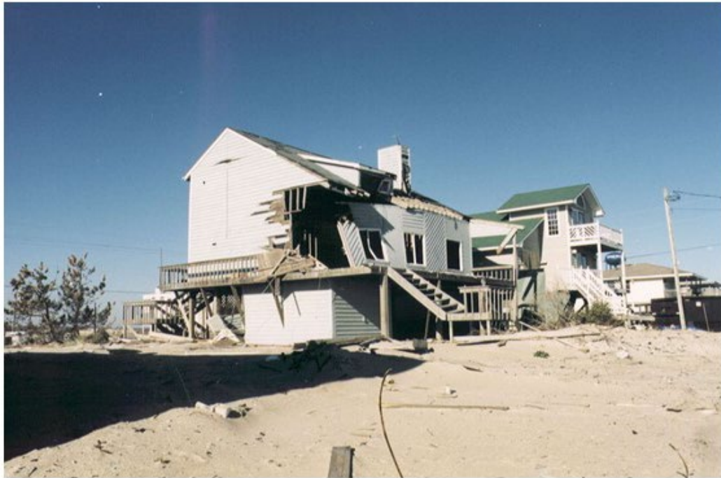
C) Wall Failure
