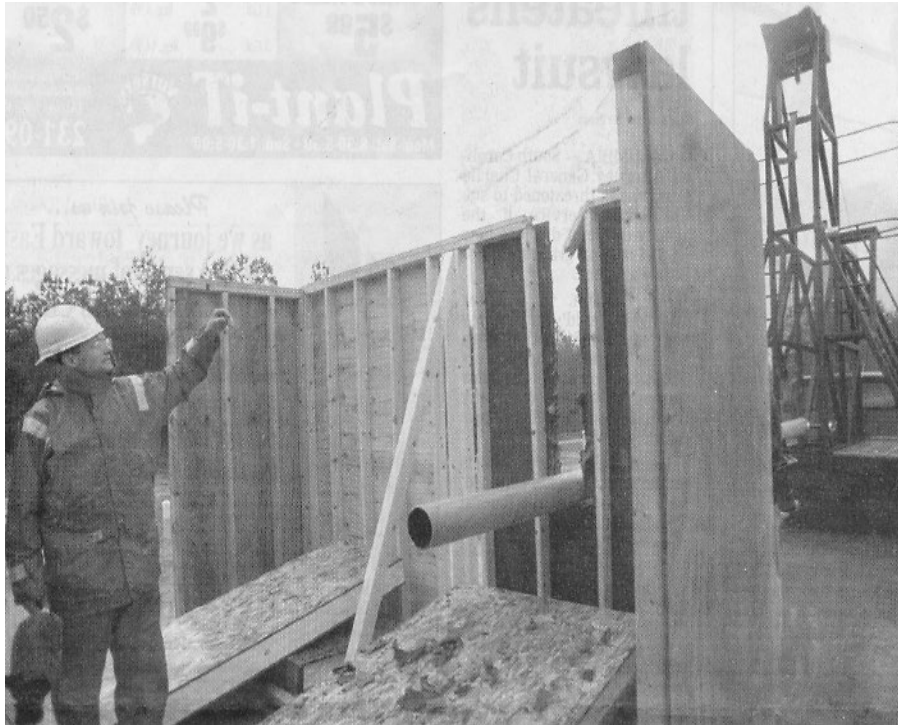
Figure 5-69 Small Pipe Impacting Wall Without Plywood Sheathing, 3,600 foot-pounds at Impact, Breaking Top Plates and Half-Way Cutting Into Wall
