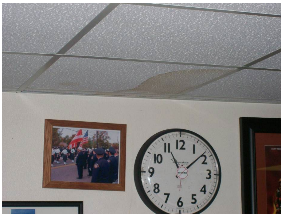
Figure 5-145 Water Damage to Interior Ceiling of a Fire Station in the Houston Area as a Result of Roof Damage (2008, Hurricane Ike)
