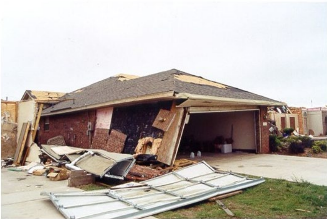
B) A wall section collapses
