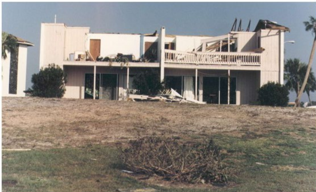
D) Whole Roof Failure, Wall Failure
