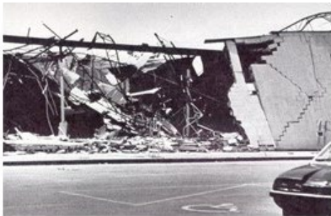
C) Collapse of masonry wall and steel frame roof system (NRC, 1991)
