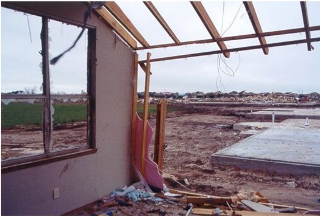
B) This photo reveals that the wall fails at nail connections to the roof and foundation
