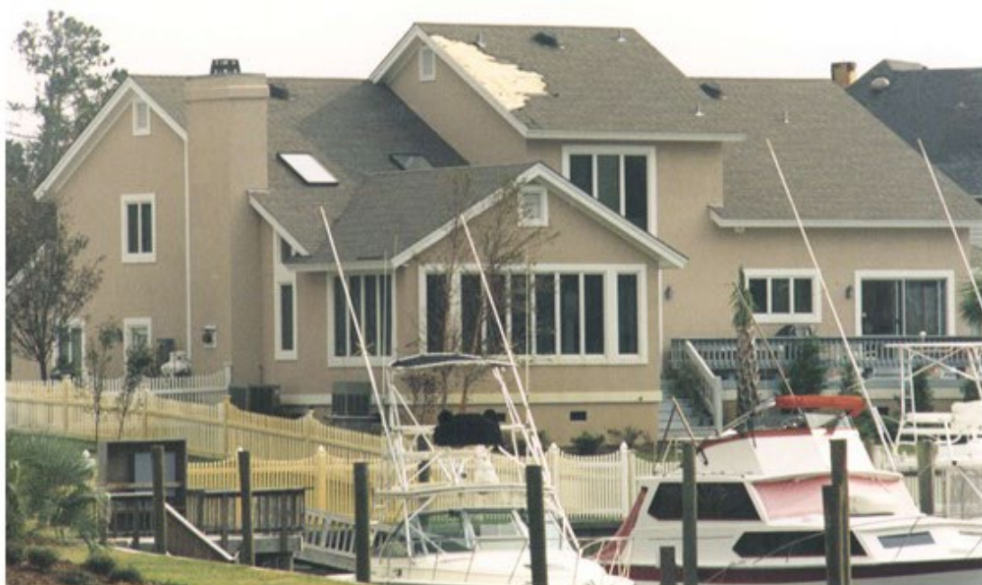
B) 2% to 15% Roof Cover Loss
