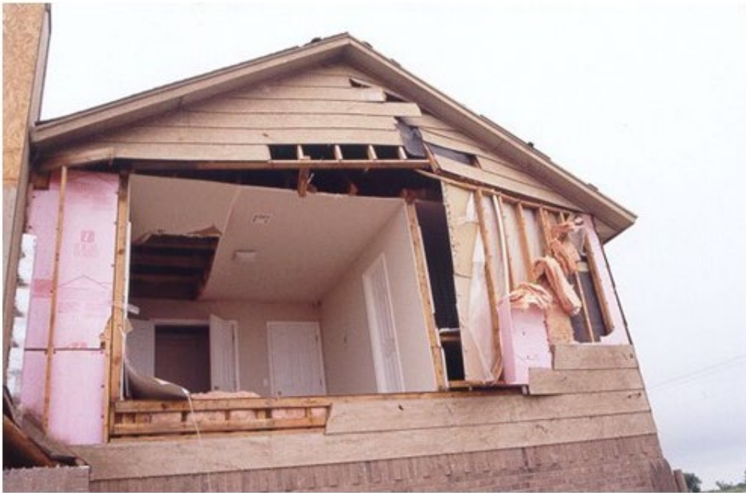
A) Exterior wall fails in sections at connections to other parts of the structure
