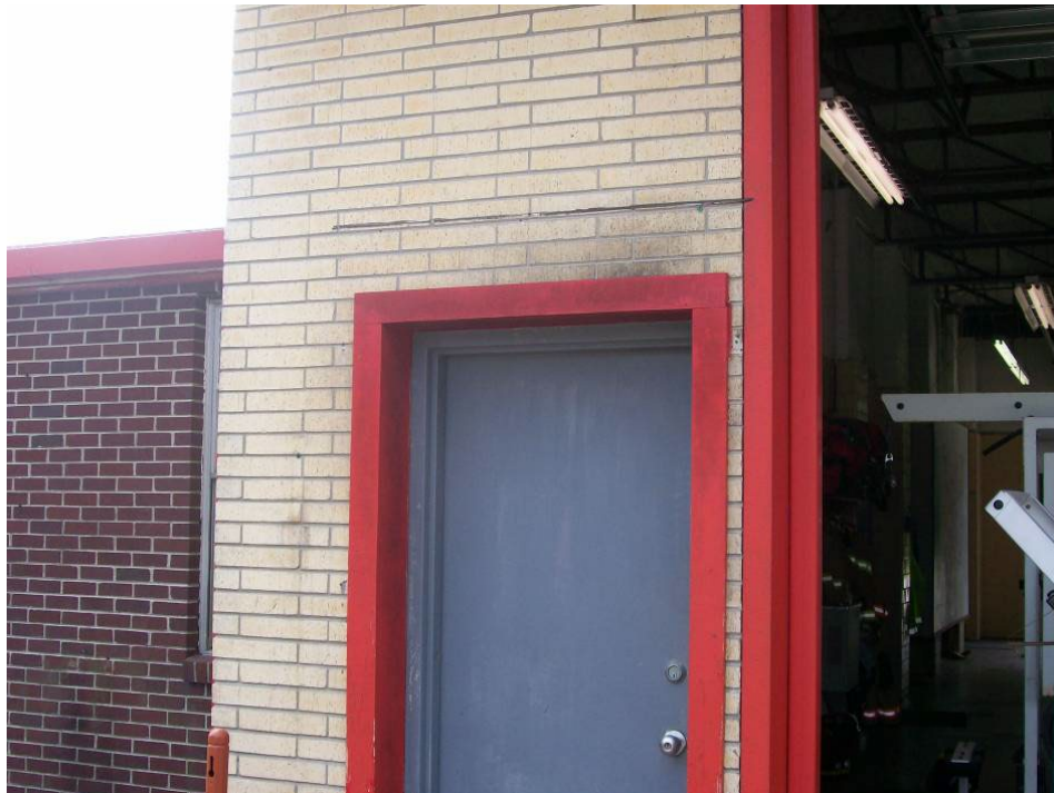
Figure 5-147 Torn Awning over Rear Entry Door for a Fire Station in the Houston Area (2008, Hurricane Ike)
