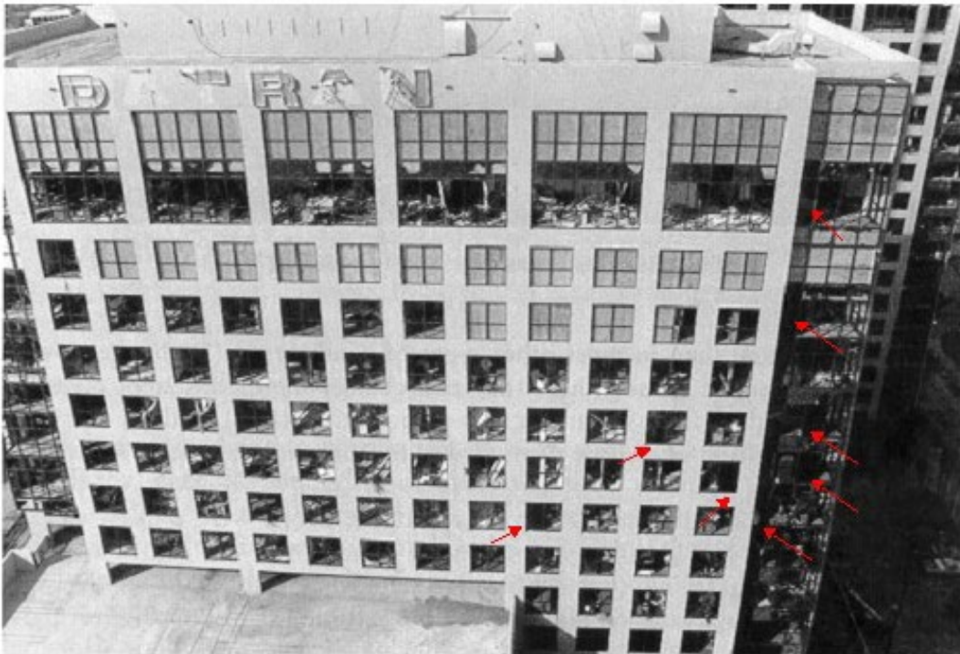
Datran Tower I, Plywood Boarding of Broken Windows Underway (Picture from Minor, 1994). Arrows indicate windows that were not damaged
