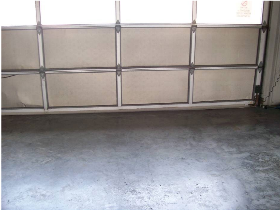
Figure 5-148 Panel Damage to Bay Doors for a Fire Station in the Houston Area (2008, Hurricane Ike)
