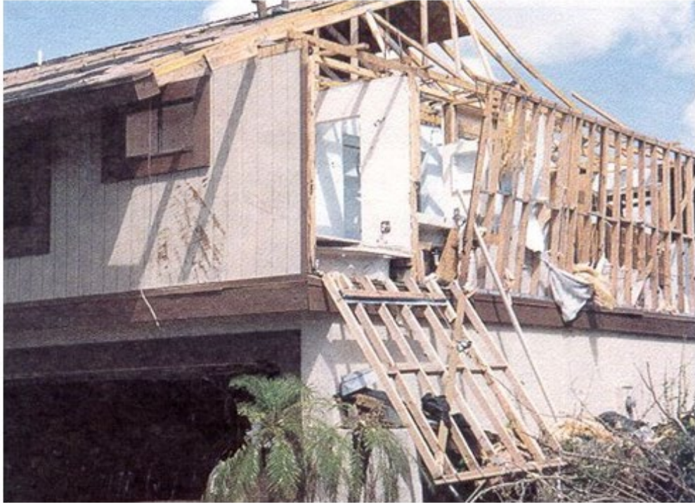
A) A let-in braced wall section collapses, while other sections also fail at connections to gable end truss
