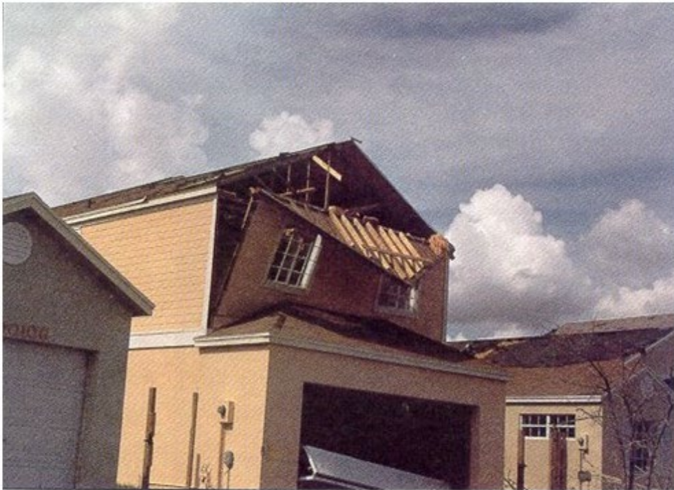
D) Another example of gable end wall connection problem
