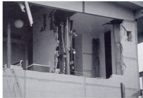
D) Collapse of masonry wall (HUD, 1993)
