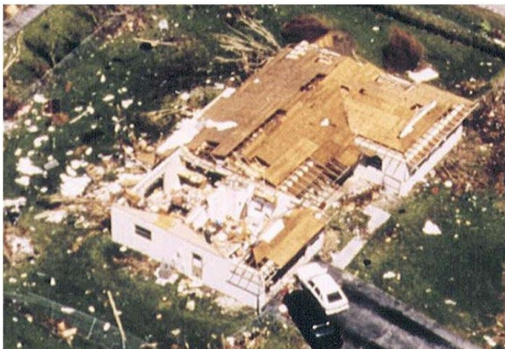
B) Complete Roof Failure, Greater than 25% Sheathing
