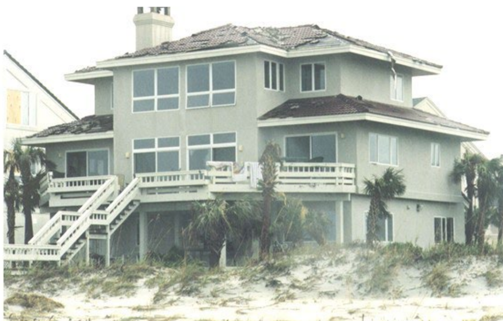
C) 2% to 15% Roof Cover Loss
