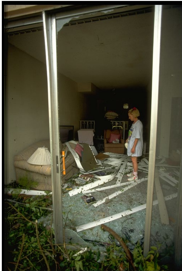
Figure 8-4 Content Losses Due to Fenestration Breach
