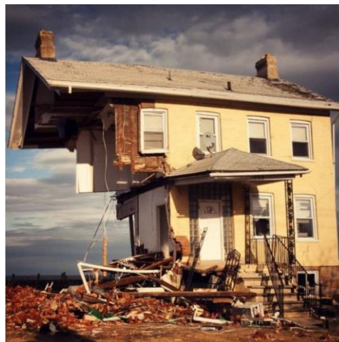
Figure 3. An example of a home sustaining major damage during Hurricane Sandy in Union Beach, N.J. in 2012.
