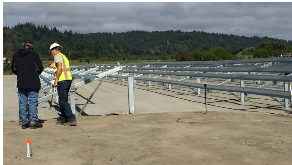
Workers installing the racking for the Blue Lake Rancheria's 500-kilowatt solar system in June 2016. The solar system is a cornerstone of the tribe's low-carbon community microgrid project.
