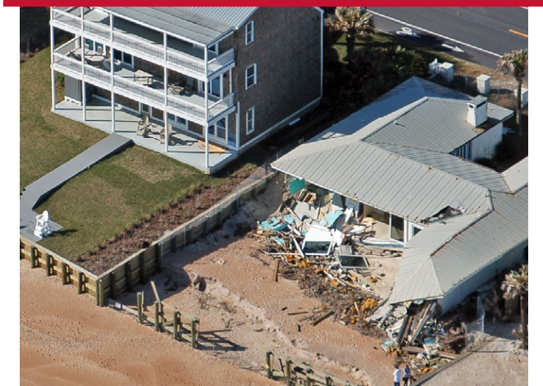
Two properties side-by-side that show how stronger building codes can protect properties
