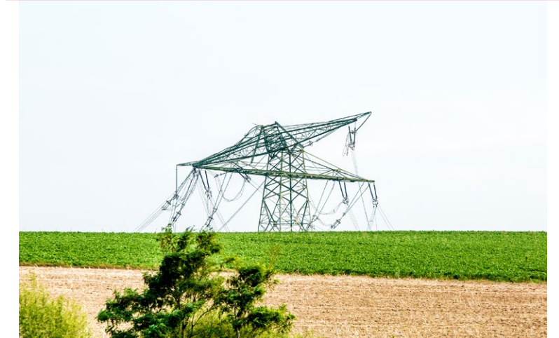
Serious storm damage on a high voltage power line after a strong storm
