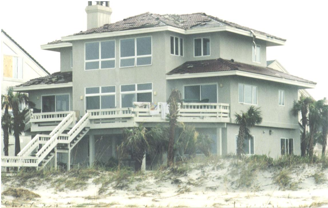
(c) 2% to 15% Roof Cover Loss
