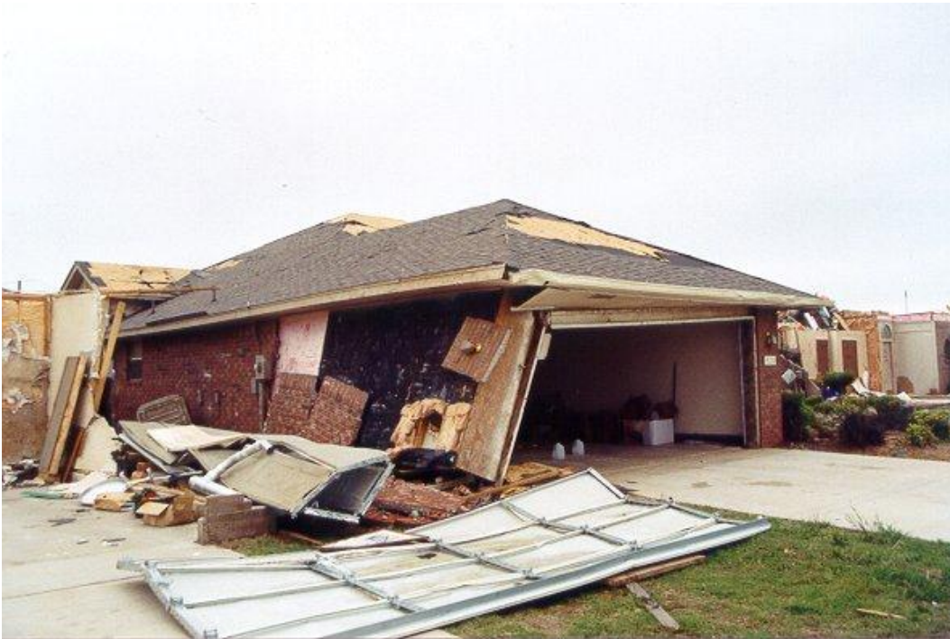
(b) Garage wall fails at the connections to the foundation
