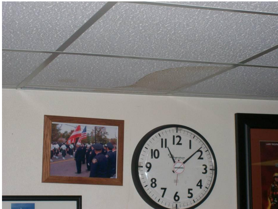
Figure 6-70. Water Damage to Interior Ceiling of a Fire Station in the Houston Area as a Result of Roof Damage (2008, Hurricane Ike) Continued.
