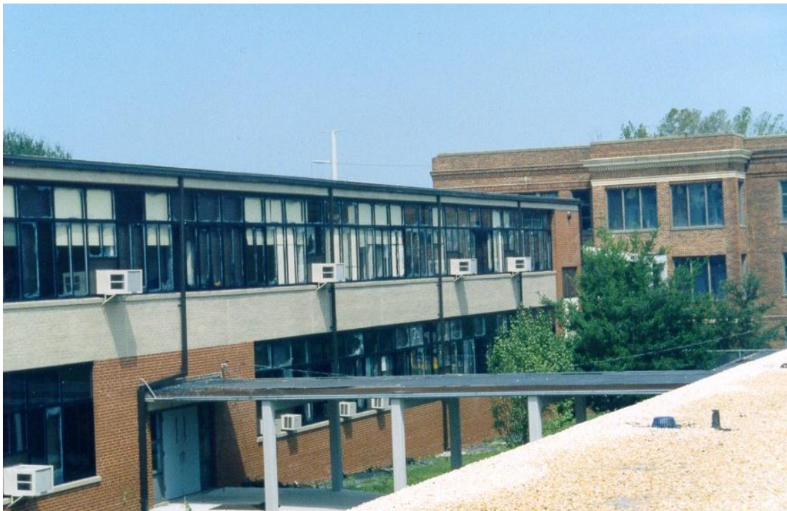
(b) Significantly Less Windows Damaged on the Lower-Right Glazed Area than on the Upper Glazed Area
