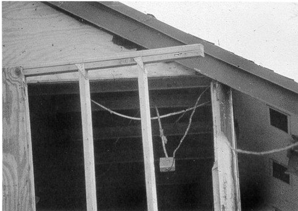
(a) Improper connection in a blown-out wall section
