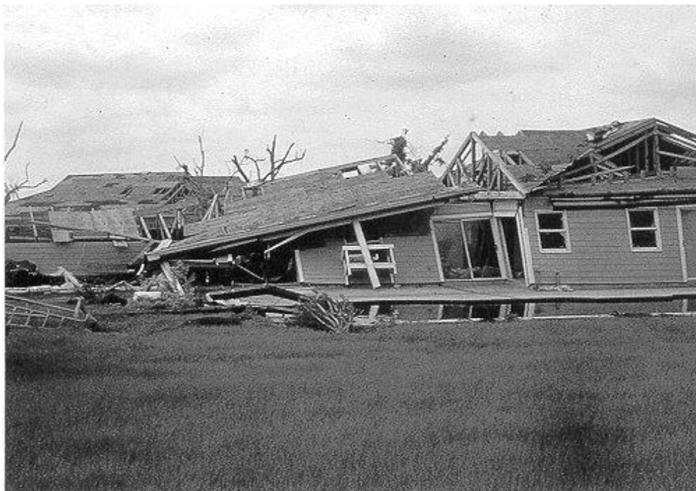
(b) Complete failure of a wood framing system
