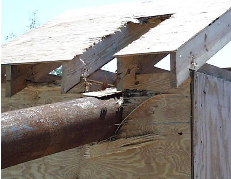
Figure 12.27. Large Pipe Impacting Roof and Wall With Plywood Sheathing, 7600 lb-ft at Impact, Breaking Roof, Top Plates and 1/8 Wall.
