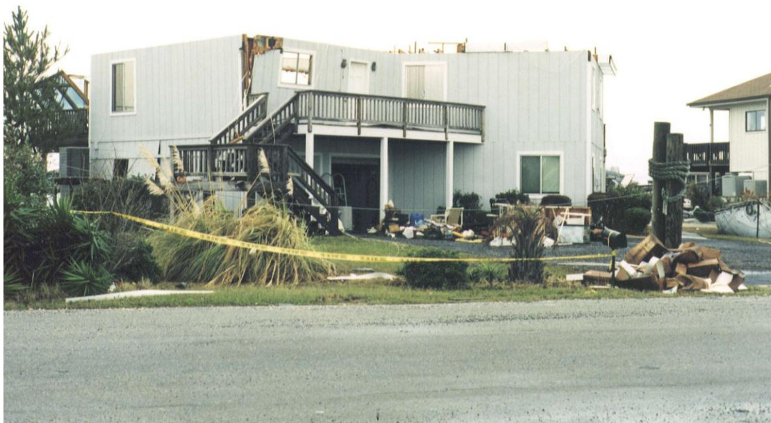
(a) Complete Roof Failure
