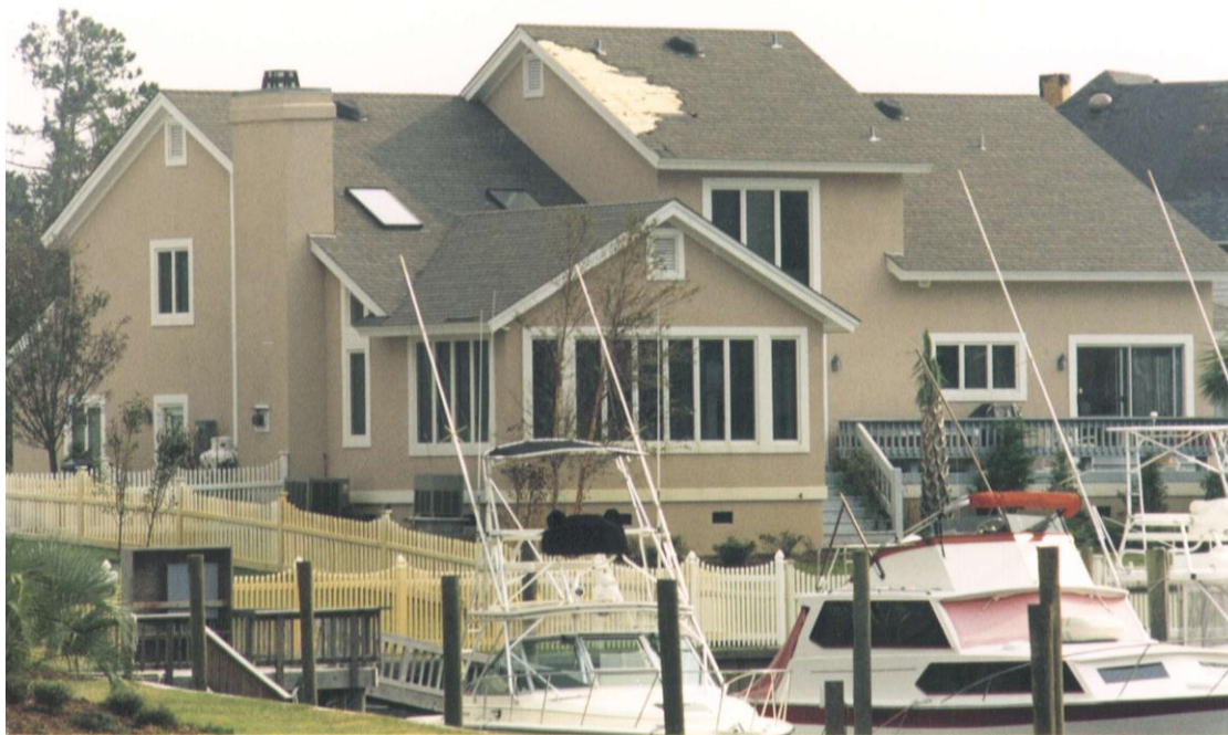
(b) 2% to 15% Roof Cover Loss
