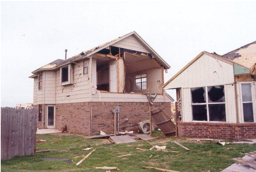
(b) Wall failure at the other side of the same building shown in (a)
