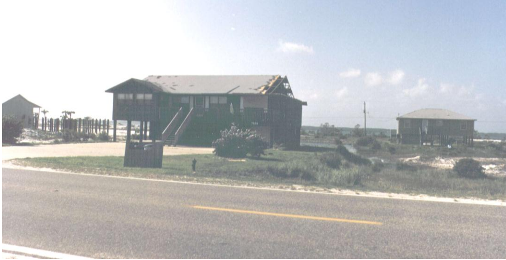
More than Three Pieces of Failed Roof Sheathing but Less than 15% of the Panels Missing
