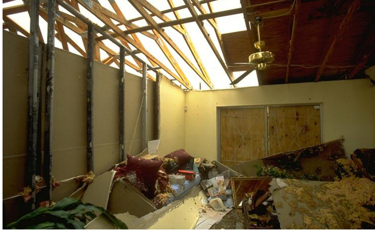
Figure 7.3. Content and Interior Losses Associated with Roof Sheathing Failure.
