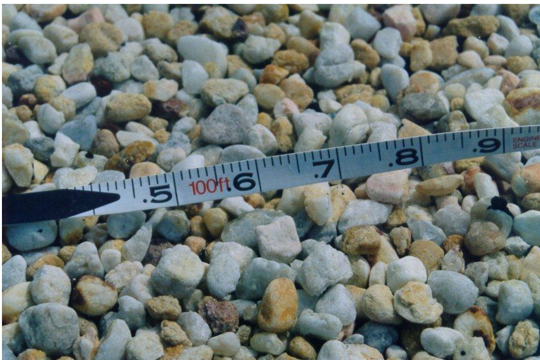
Figure 5.18. Roof Gravel on the Upstream Building.
