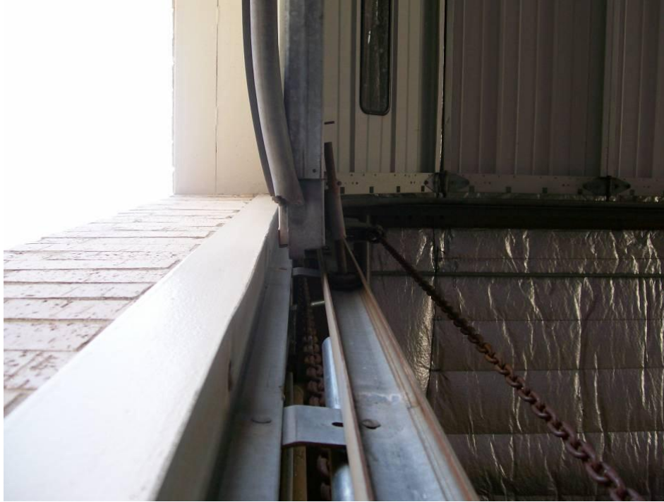
Figure 6-71. Bent Bay Door Rollers for a Fire Station in the Houston Area (2008, Hurricane Ike).
