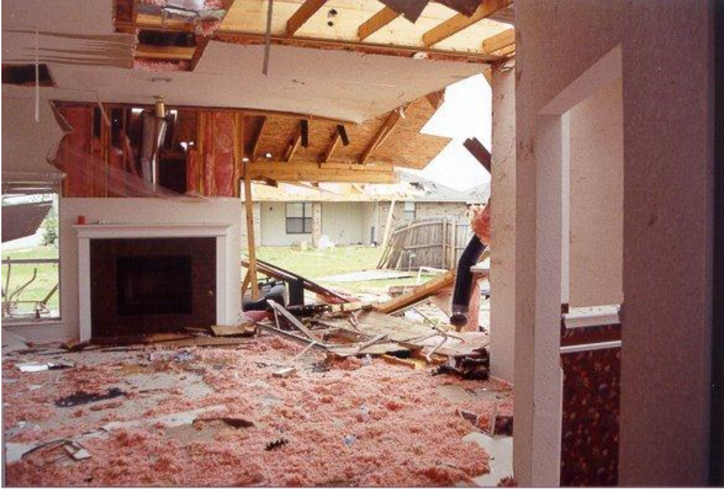
(a) A wall section collapses
