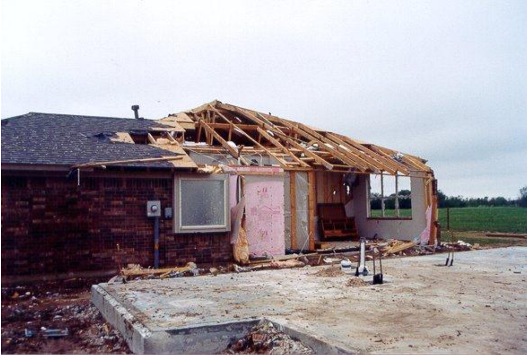
(a) Wall failure while roof frame still in place
