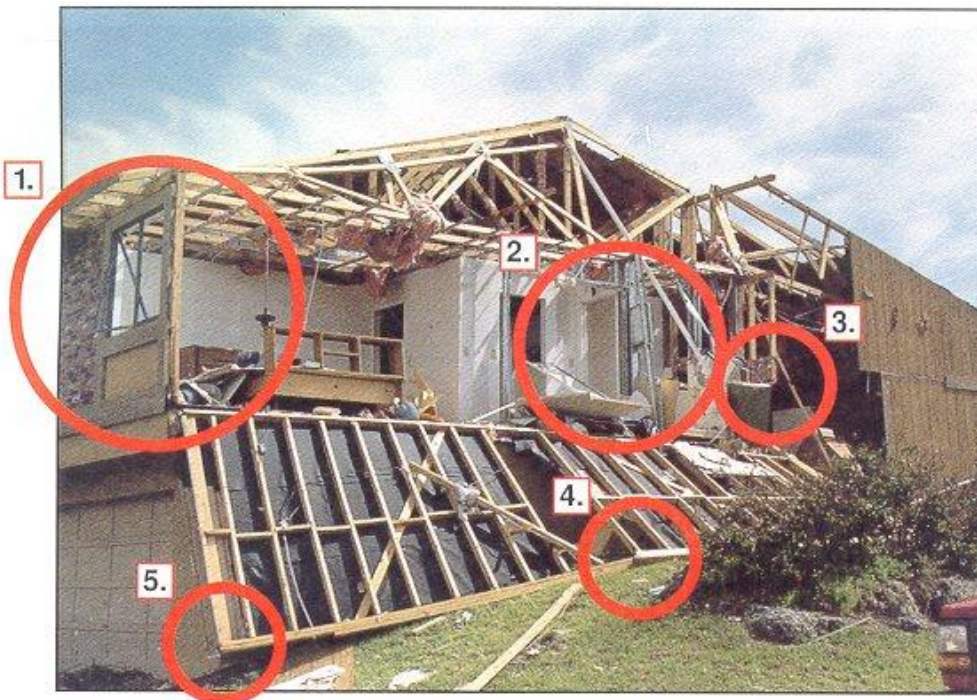
(b) Several sections of a let-in braced wall collapse, failed at connections to gable end truss
