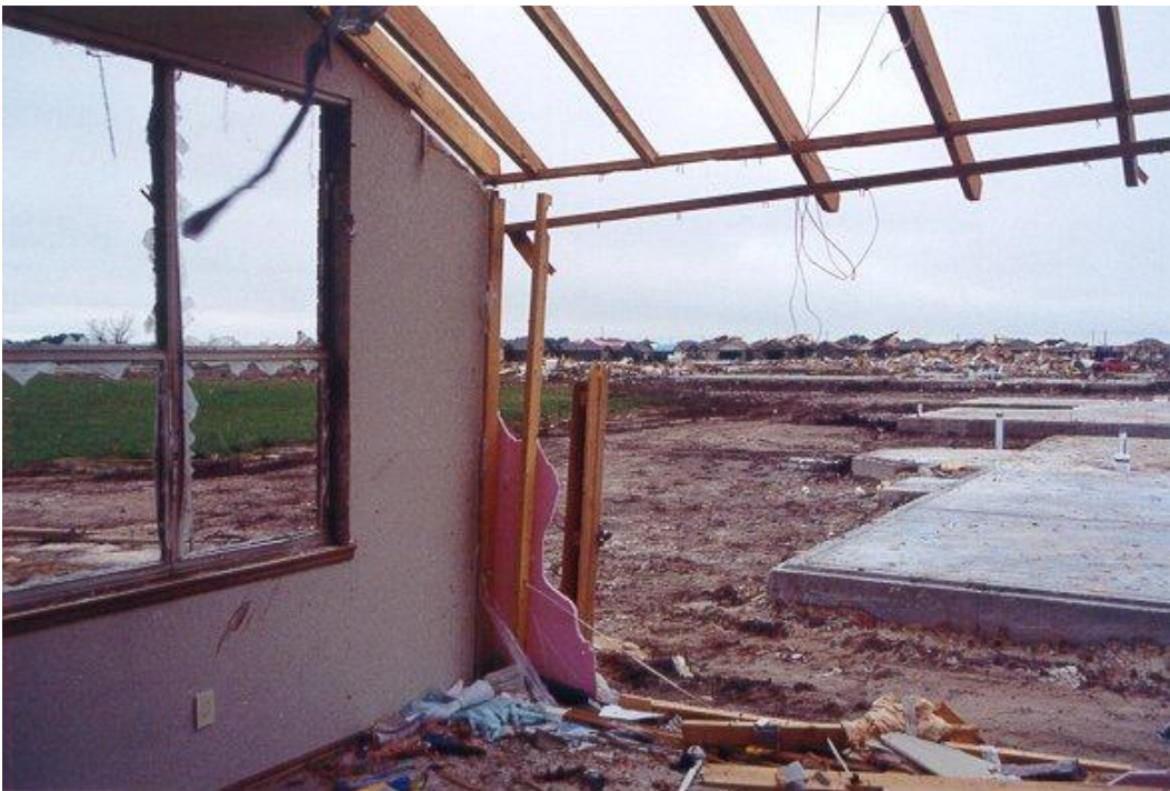
(b) This photo reveals that the wall fails at nail connections to the roof and foundation
