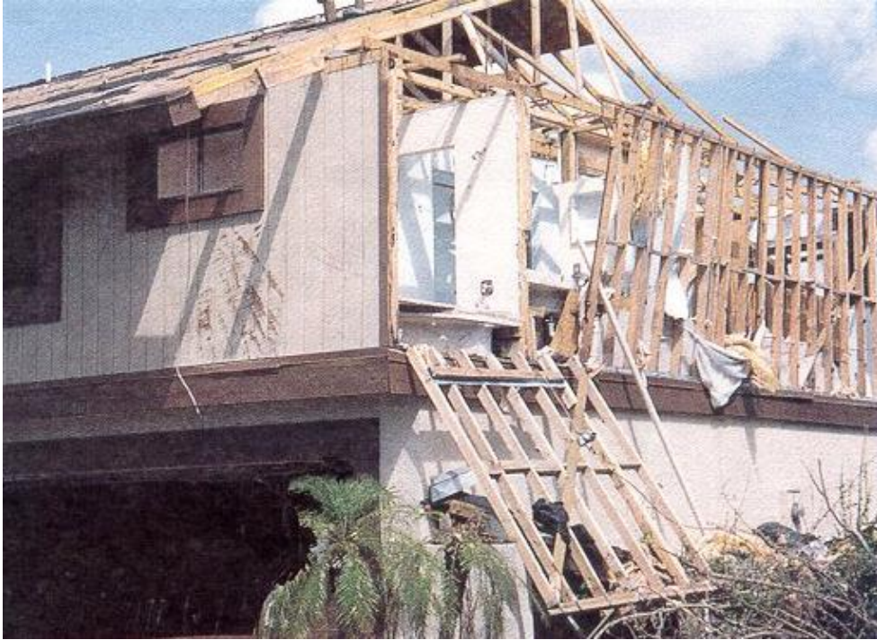
(a) A let-in braced wall section collapses, while other sections also fail at connections to gable end truss
