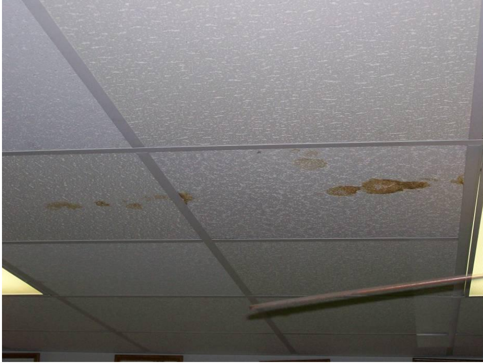
Figure 6-69. Water Damage to Interior Ceiling of a Fire Station in the Houston Area as a Result of Roof Damage (2008, Hurricane Ike).
