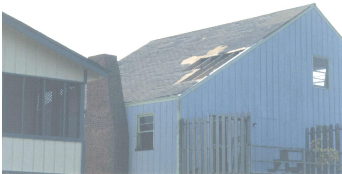
(b) At least One Failed Sheathing but Less than Three Failed Pieces of Roof Sheathing
