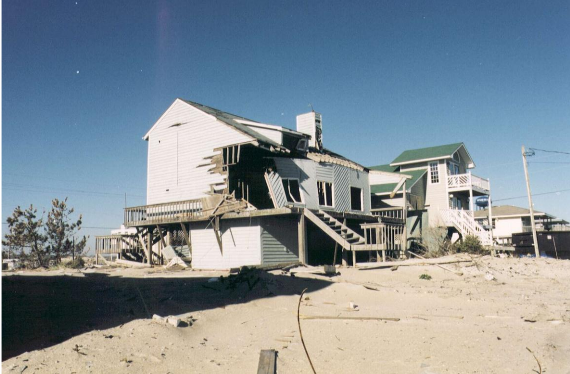
(c) Wall Failure
