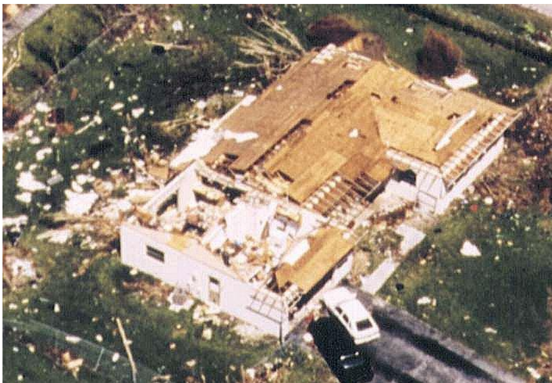
(b) Complete Roof Failure, Greater than 25% Sheathing
