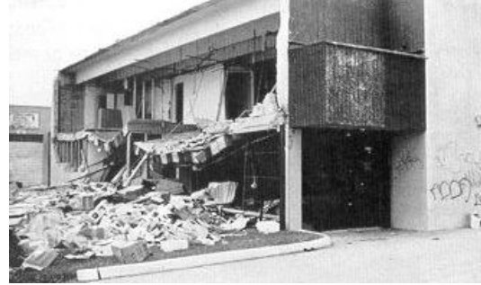
(b) Collapse of masonry walls (Zollo, 1993): A wall of 40' span (top); Walls on a two-story building (bottom)
