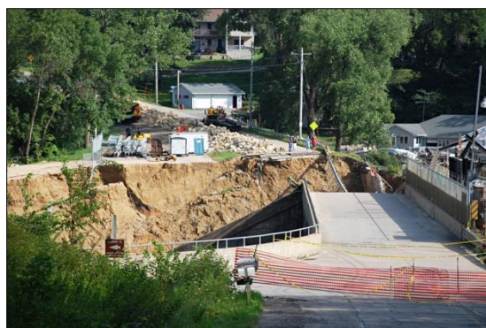
Collapse of Lake Delhi Dam (Iowa) in 2010 severed a road
