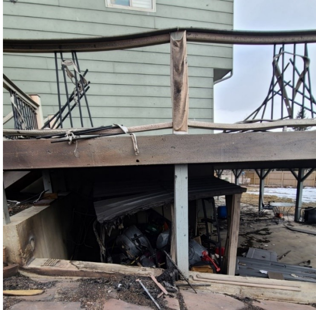
Figure 49. Elevated decks and concrete patios attached to homes were commonly observed. Many elevated decks had combustible materials stored beneath them.
