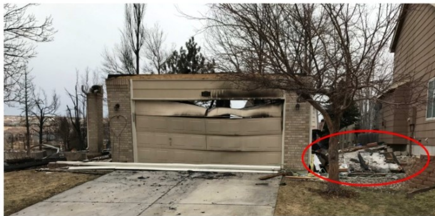
Figure 55. Sample evidence of combustible fencing attached directly to single-family residences in Louisville, Colorado, and serving as a fire pathway to an adjacent home.
