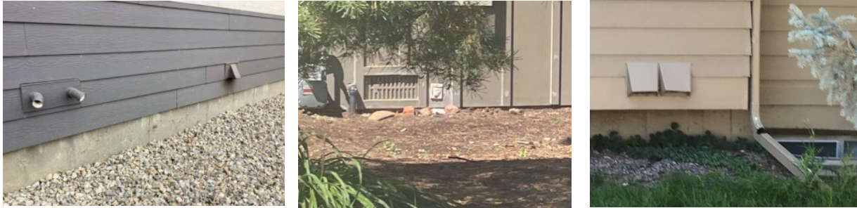
Figure 43. Lack of vent protection in exterior walls, crawlspaces, and basements in Superior and Louisville, Colorado.
