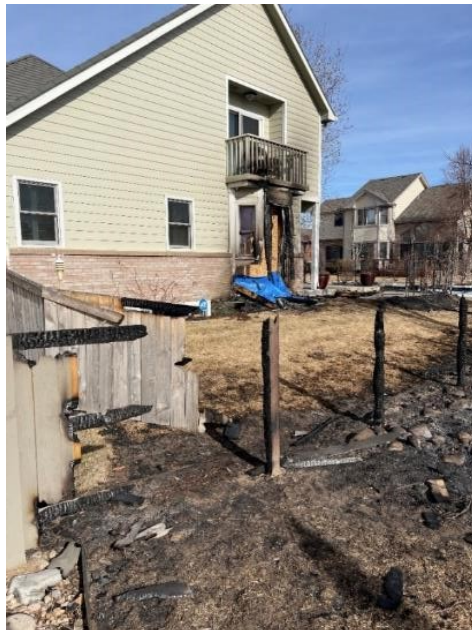
Figure 51. Balconies can catch on fire from below, which can result in spreading fire to upper levels of the house.
