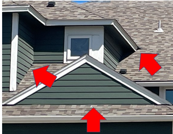
Figure 32. Example of observed areas where use of metal flashing could provide additional protections.
