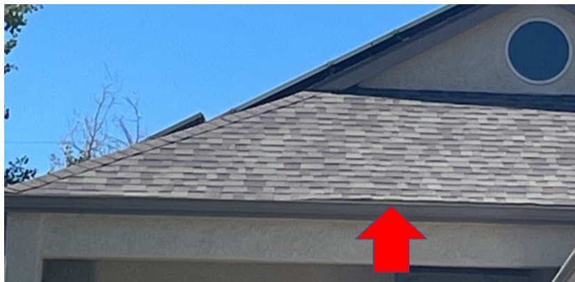
Figure 36. Example of observed vulnerable areas where metal flashing could provide additional protection.
