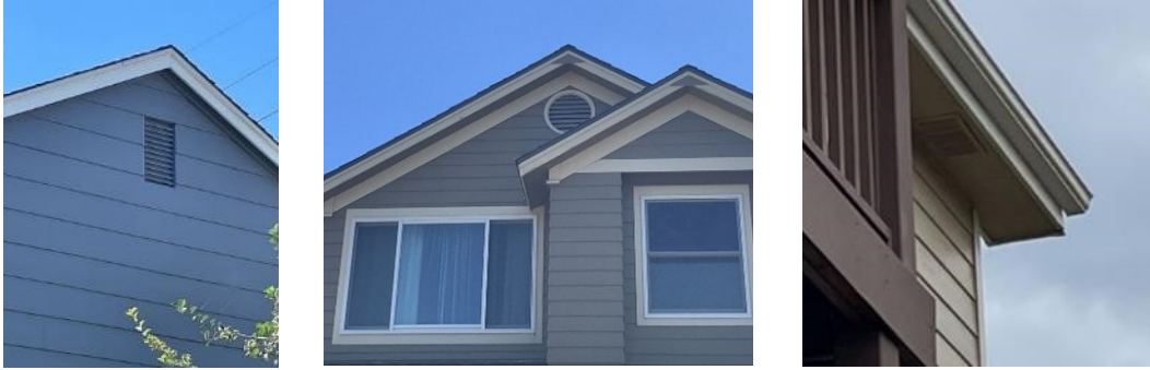
Figure 27. Lack of vent protection in attic vents, gabled roof attics, and soffits in Superior and Louisville, Colorado.
