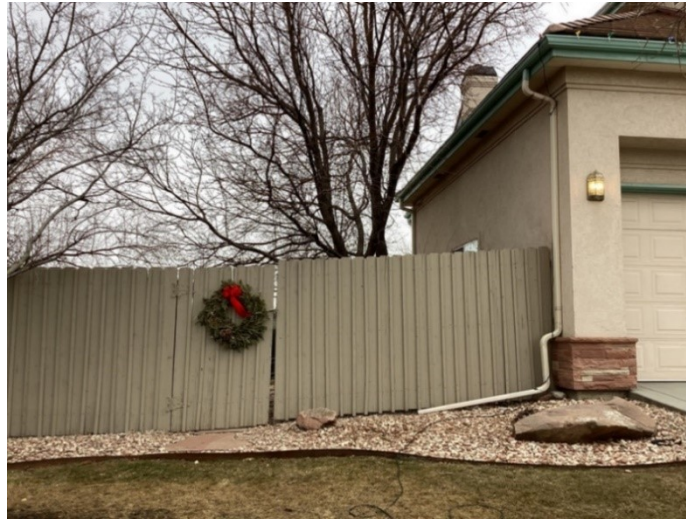
Figure 52. Combustible fencing directly attached to a single-family residence in Rock Creek Ranch in Superior, Colorado.
