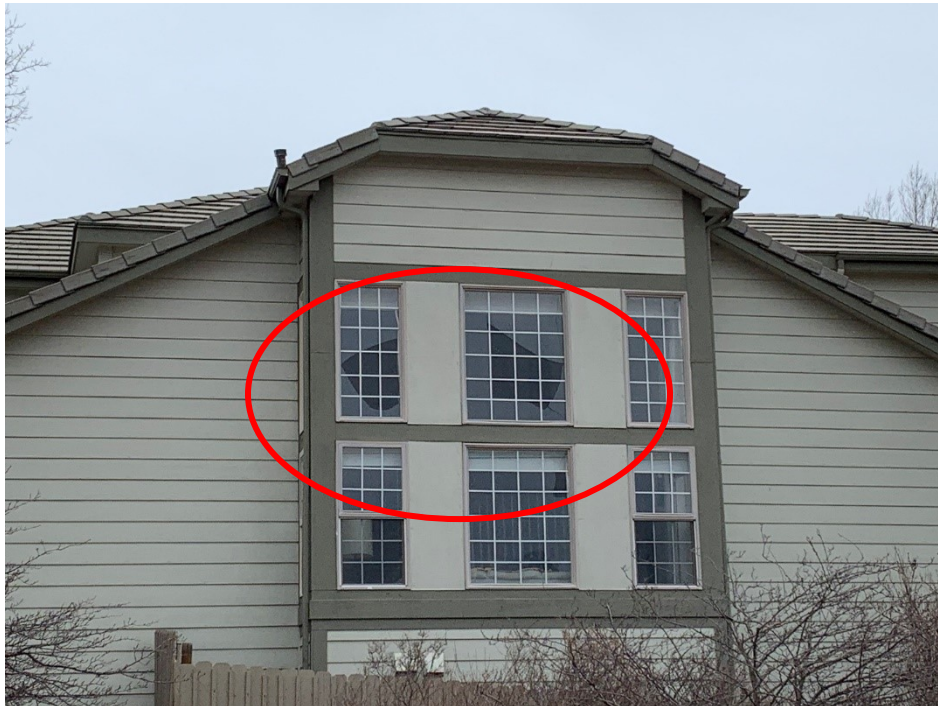
Figure 41. Some multi-pane windows showed evidence of the outer glass breaking.
