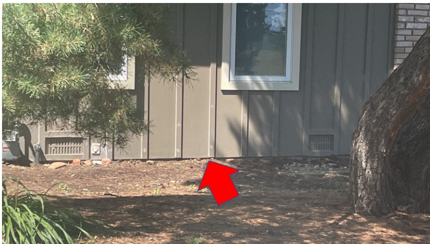
Figure 46. Example of a home without adequate bottom-of-wall clearance.
