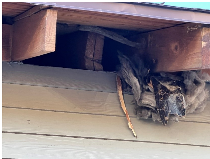
Figure 28. Wood blocking or attic vents blow out possibly due to high winds.
