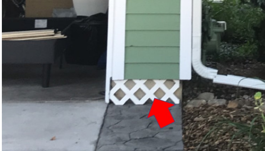
Figure 47. Example of home provided with adequate bottom-of-wall clearance but with obstructions.
