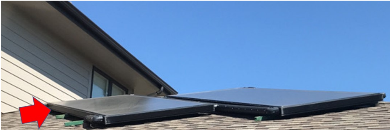
Figure 29. Example of observed unprotected solar panel installation.
