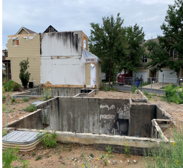
Figure 42. A Marshall Fire-damaged townhome built in 1998 in Superior with tenant separation wall not extending to underside of roof sheathing.
