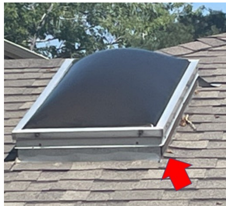
Figure 34. Example of metal flashing at joint between the skylight unit and the roof.
