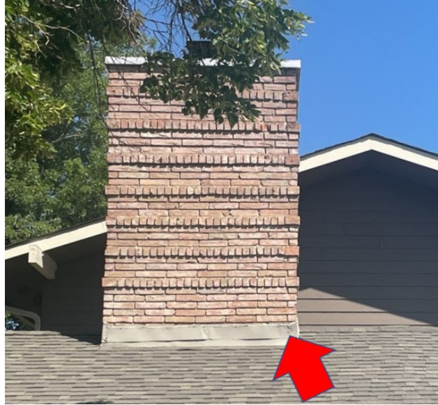
Figure 33. Example of observed gaps at chimney-to-roof joint.
