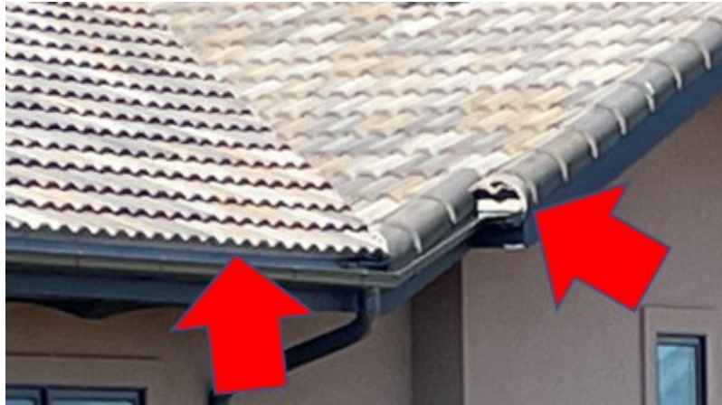
Figure 35. Example of observed profile-tiled roof with gaps at the roof edge.
