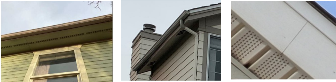
Figure 37. Observed vent protection for soffit eave vents in Superior and Louisville, Colorado.
