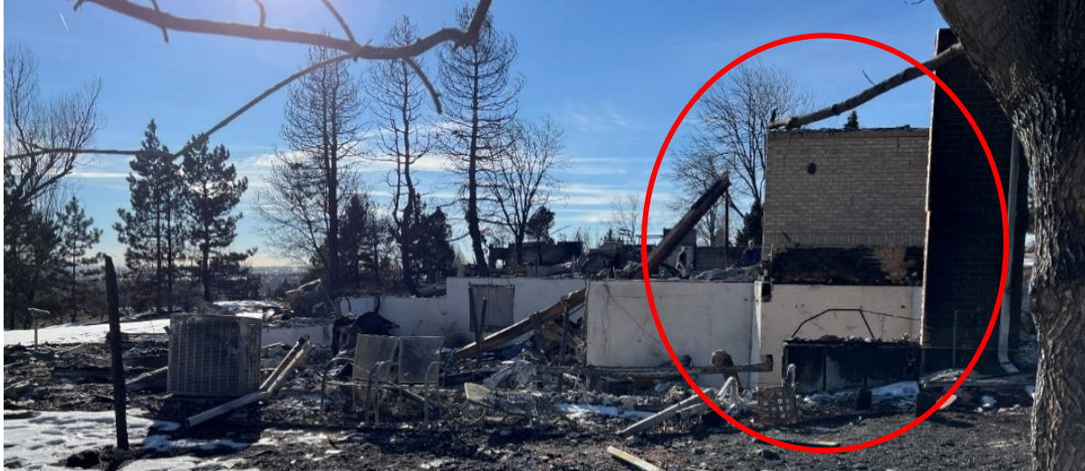
Figure 38. While blackened by smoke, soot and ash, concrete and brick elements remained standing more often than most other exterior wall construction materials.
