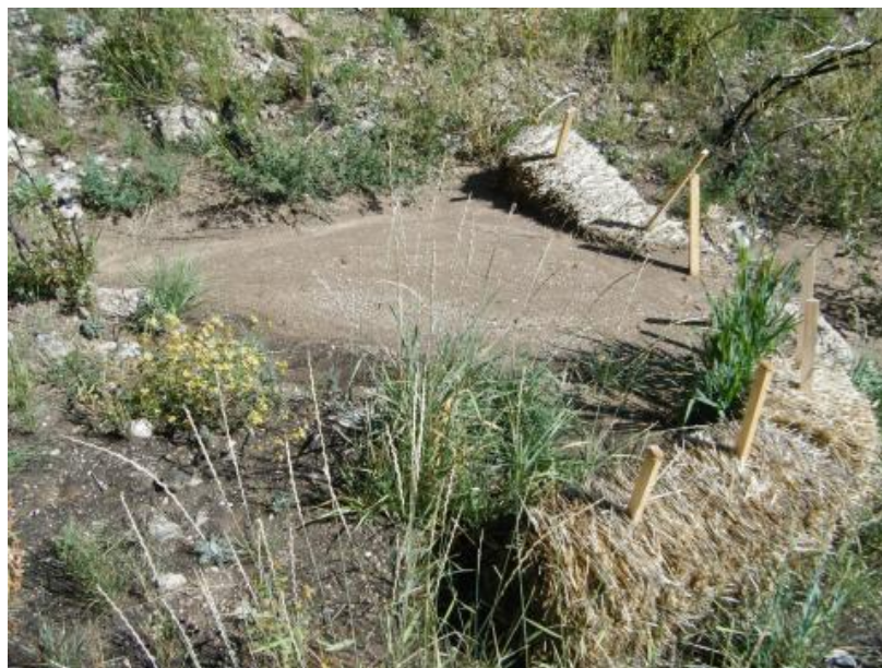
Figure 17. Straw bale check dams can reduce post-fire runoff from steep channels by capturing sediment during rainfalls (USDA Forest Service photo by Pete Robichaud, n.d.).
