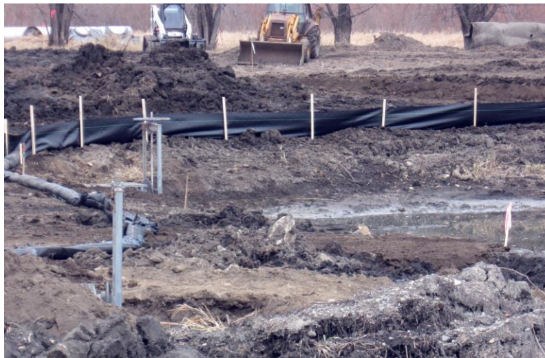
Figure 15. Silt fences and mulch can help prevent erosion after a wildfire (Gerry Shimek, USFWS, n.d.).
